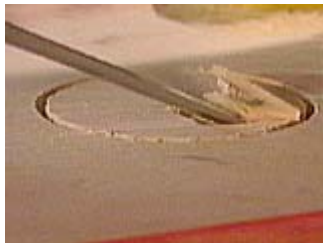
Chisel the wood out to the depth cut by the hole saw
