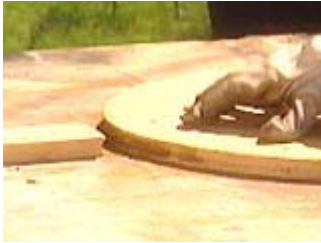
Attach two pieces of wood to a table top as a jig to bend the re-bar
