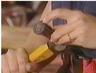
Using a framing hammer with a waffle face makes driving nails easier
