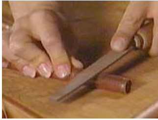
To drill the holes, first file a little flat spot on the pipe
