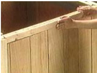
Cut the doors to fit inside the trim and one half to one inch off the ground
