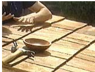
Determine the shingle exposure by measuring and dividing the roof top distance
