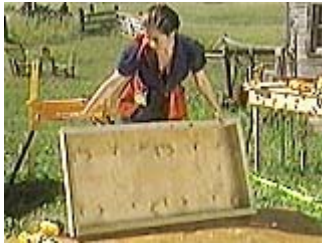
Make a floor out of pressure treated 2x4 and exterior grade half inch plywood
