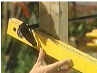
Clamp a straight edge on the front post and experiment with the roof pitch
