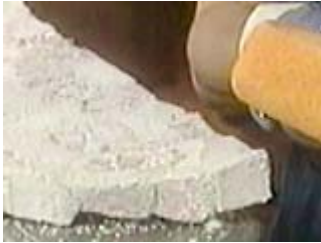
Use a tile sponge with softened edges and corners to clean off the excess grout
