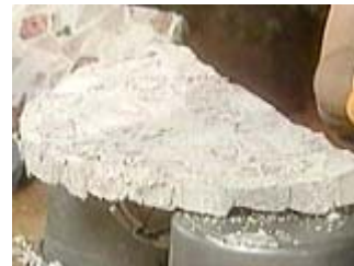
Fill all the spaces - use your finger to press it in if necessary
