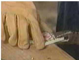
Use pliers to break the tile down and away from the cut line
