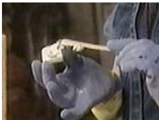
Put more mortar on the thin pieces so that the tops become level
