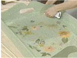
Install some clear silicone dots to help support the glass along the edge
