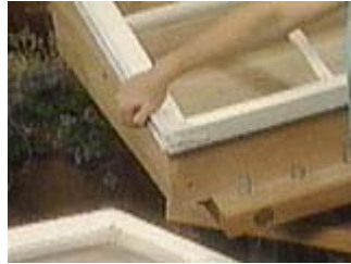
The box will be smaller than the window so that the rain will drip off
